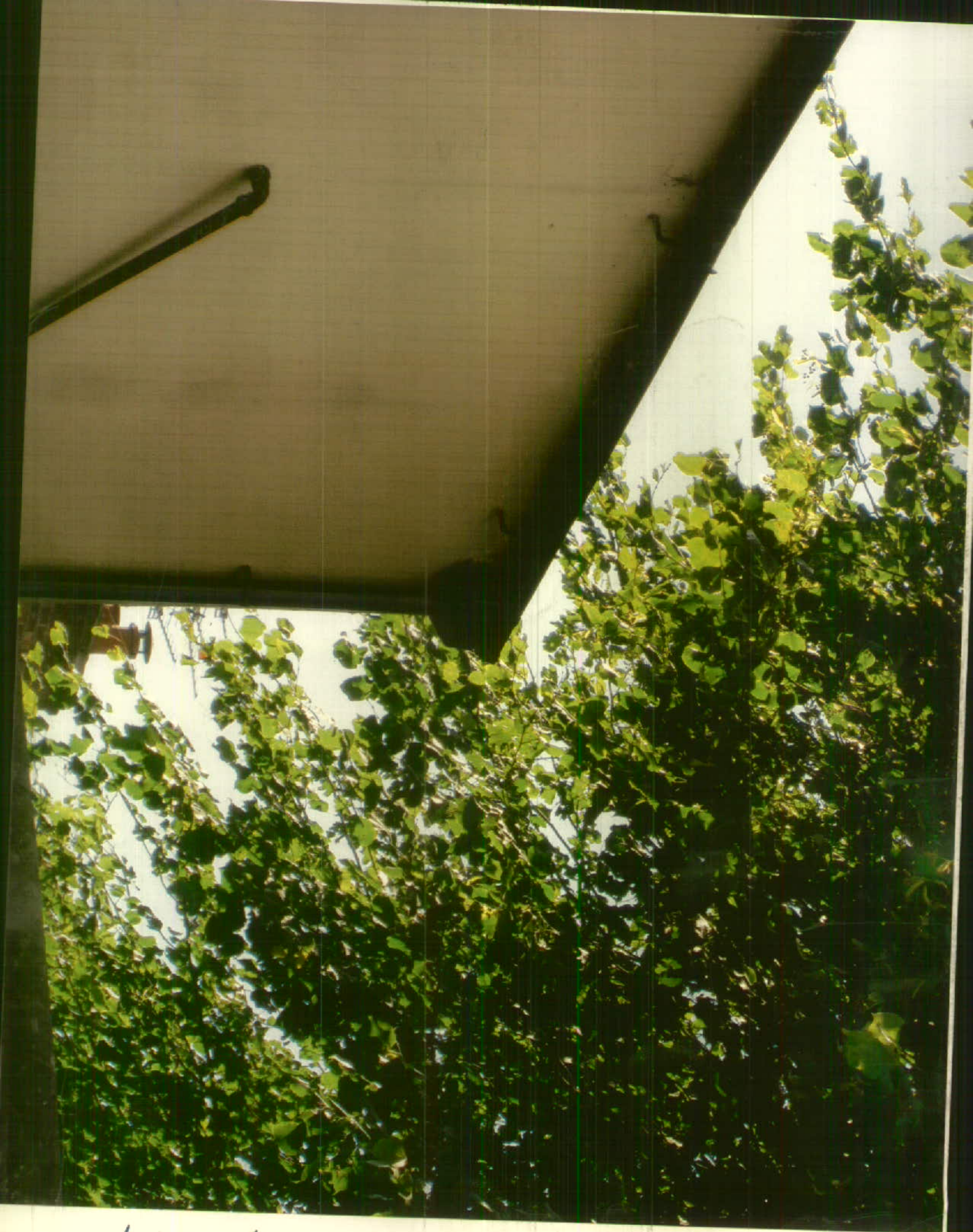
lower branches striking roof and wall at the house! Photo 5
