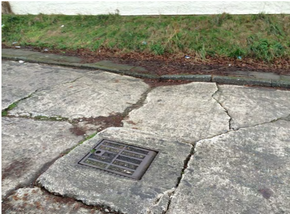
Figure 11: Collapsed drain in access road to south of buildings.
